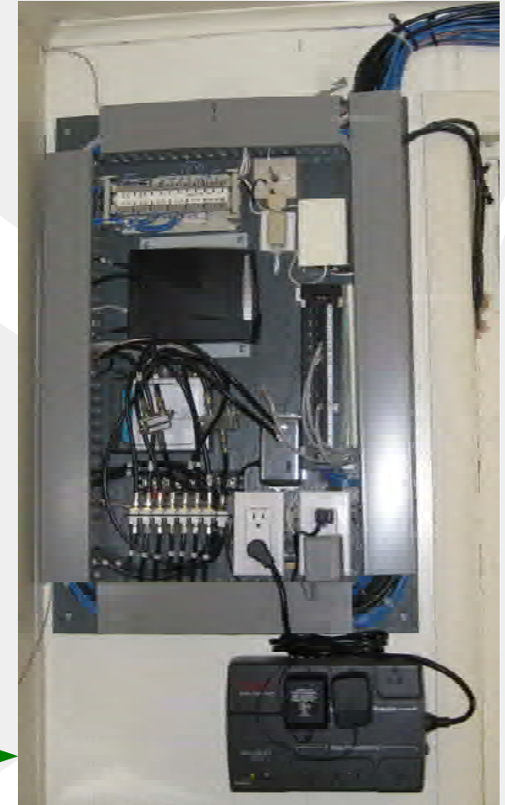
Multimedia Patch Panel in basement Phone, Video, Network, CCTV, Audio
